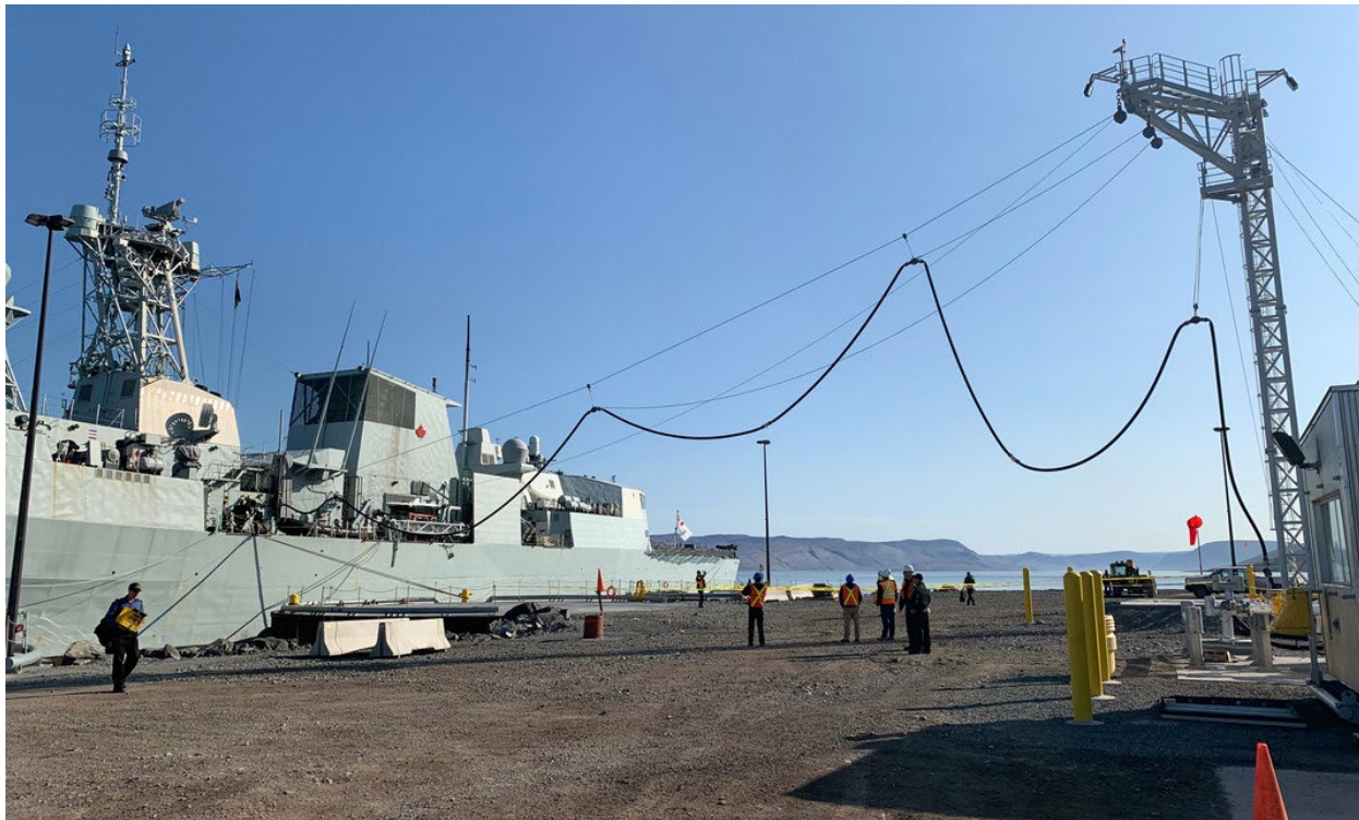
Figure 11: Spanwire Supported Fueling (SSF) system during 2019 visit of HMCS Ville de Quebec . Photo credit: Stoker. Nanisivik Naval Facility 17 October 2019 at https://army.ca/forums/threads/nanisivik-naval-facility.130989/ .
