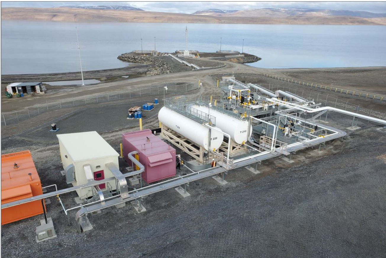
Figure 12: Operational Area (Gensets, POL storage, Diesel tanks, Pump platforms). DCC, “Nanisivik Naval Facility (NNF) Construction 2022 Annual Report Revision 1,” 15 November 2023.
